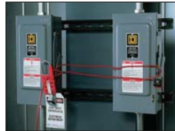
Lockout single or multiple electrical disconnects
