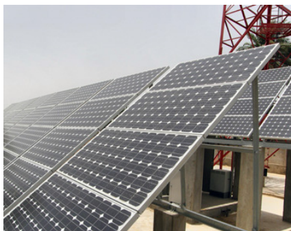
Solar-powered Cellular Base Station
