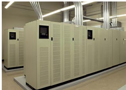
Uninterrupted Power Supplies
